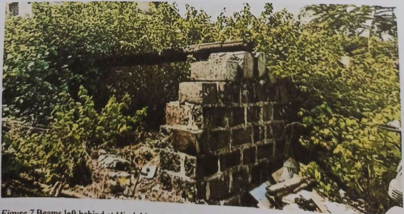
Figure 7 Beams left behind at Hiralal Leather Works
